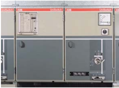
Low voltage compartment
